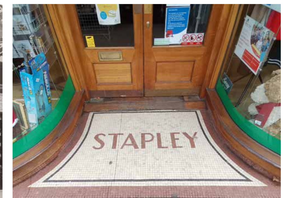
Mosaic paving tiles to the Stapley building entrance on the High Street (present day).
